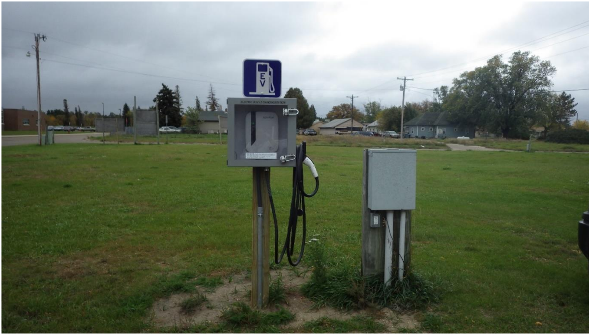
Figure 3. EV charging station at the Red Lake Department of Natural Resources, installation complete 8/3/2020.
