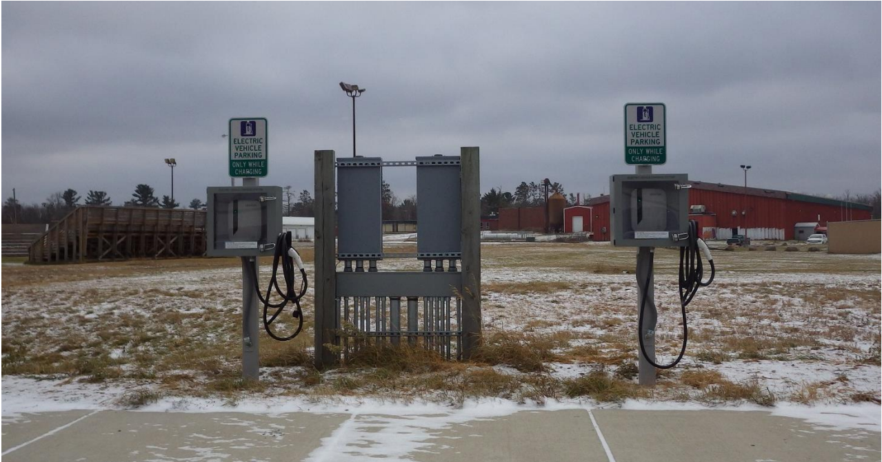
Figure 1. EV charging stations at the Red Lake Nation College, installation complete 8/3/2020.
