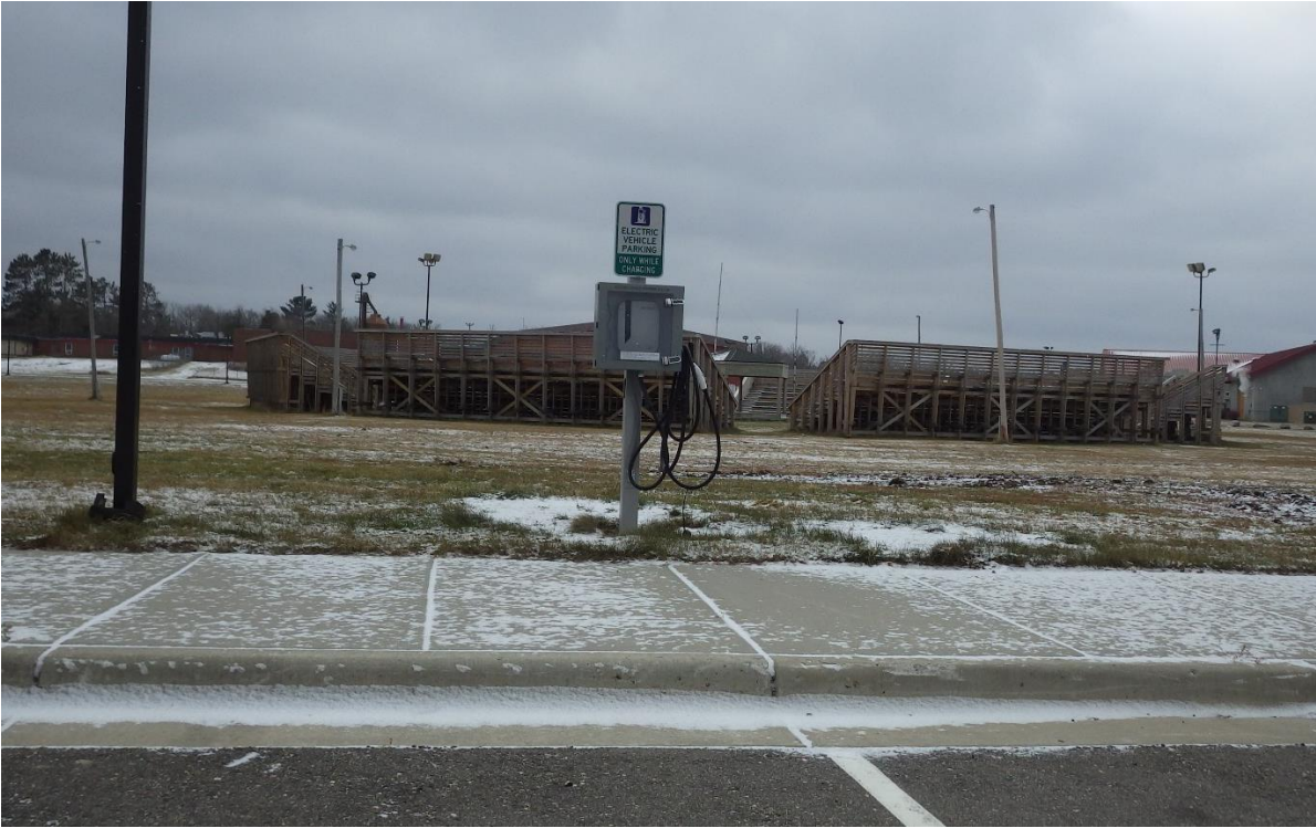
Figure 2. EV charging station at the Red Lake Government Center, installation complete 8/3/2020.
