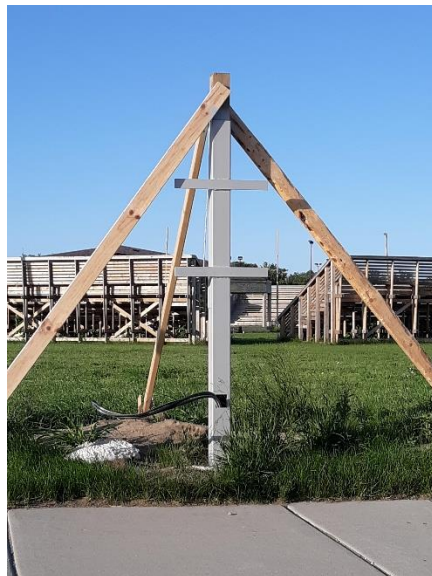
Figure 4. EV charging station at the Red Lake Government Center (installation not complete).
