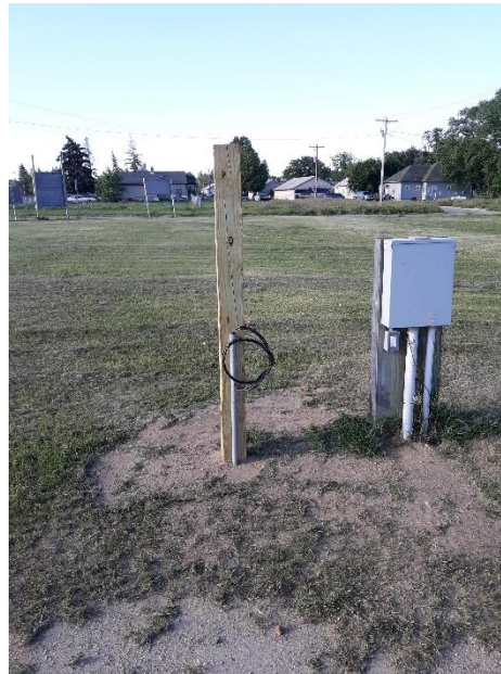
Figure 5. EV charging station at the Red Lake Department of Natural Resources (installation not complete).
