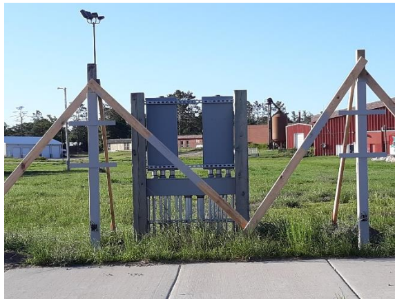
Figure 3. EV charging stations at the Red Lake Nation College (installation not complete).
